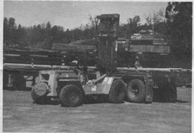
Day 40. A truck arrives with the structural skeleton of our soon to be completed building.
